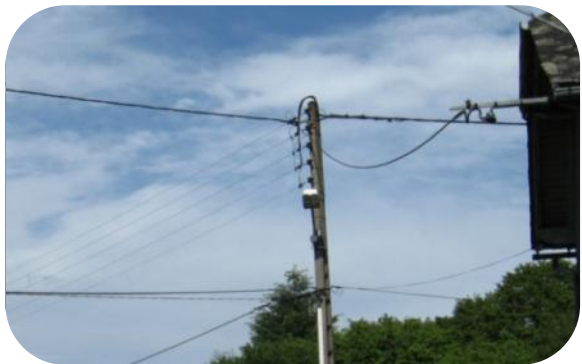
Lignes BT (basse tension) 230/400 volts
